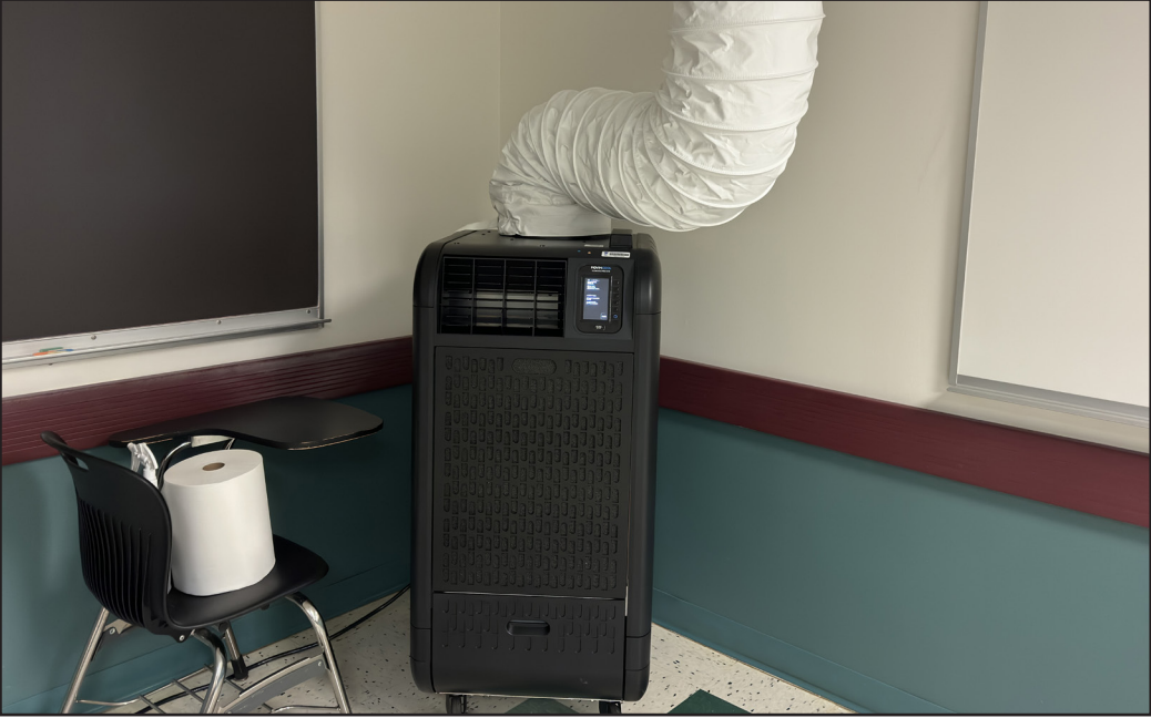
Air conditioning in Room 014 in Morrill Hall.
